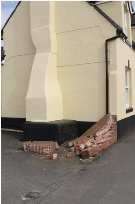
The collapsed wall at No 53 High Street. You can see that it was hit pretty hard.
